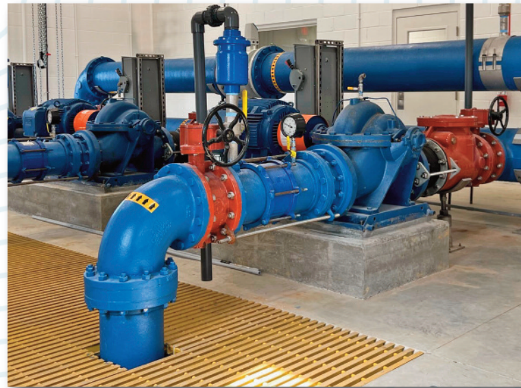
The Route 40 Booster Station enables Artesian to push available water supply from southern New Castle County to northern New Castle County, reducing our purchased water expenses with Chester Water Authority.
