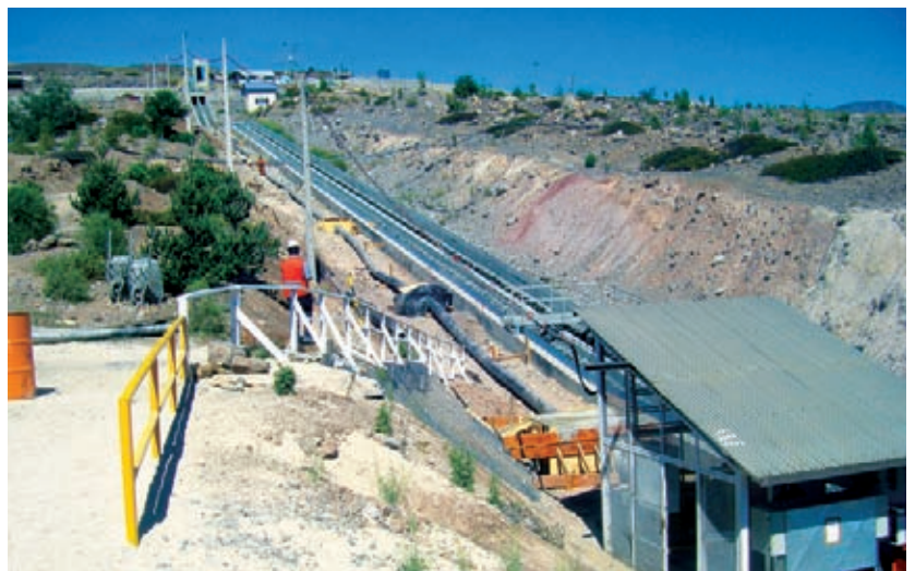
Pumping station at Codelco's El Teniente copper mine in Chile
