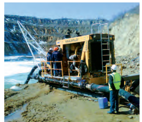
A dewatering solution from Weir Minerals Multiflo in Amurskaya, Russia
