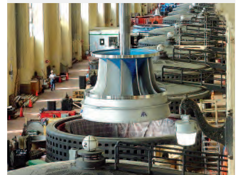
Keokuk Hydroelectric Station, USA
