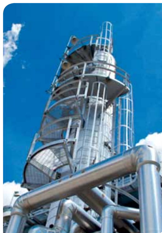
Gas Fractionation Tower
