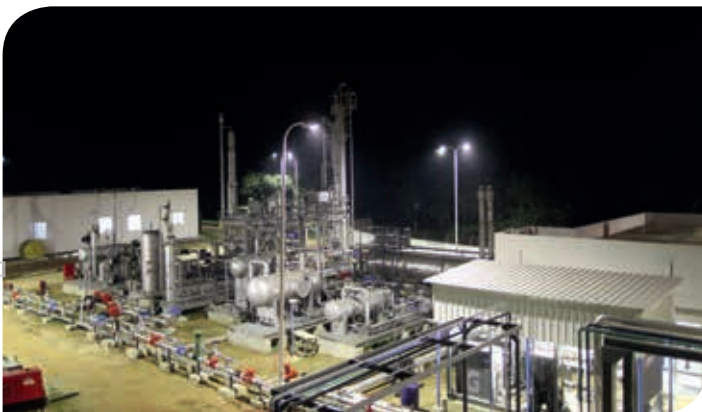
30MMSFD TEG Gas Dehydration Plant
