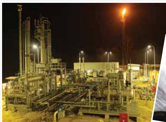
Gas Processing Plant
