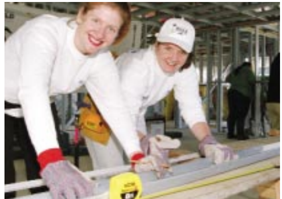
VOLUNTEER TEAMS OF WOMEN WORK TO BUILD AFFORDABLE HOUSING IN WESTERN SYDNEY USING STEEL FRAMING MADE FROM ZINCALUME® STEEL.
