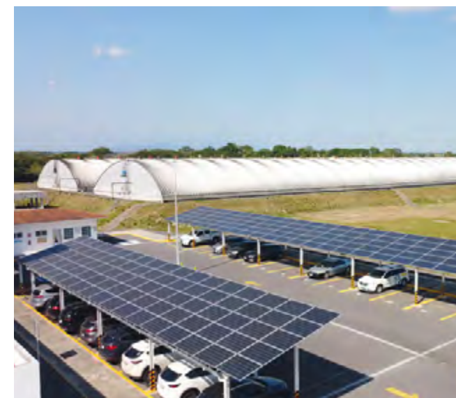
AB Mauri's Veracruz site, in Mexico, installed 205 solar panels, which generate half of all the energy used by their site offices.
