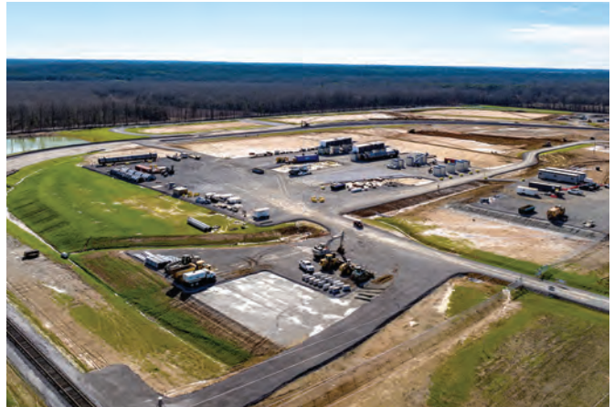
► Biocarbon Production Facility | Photo: Mike Hainsey, Northstar Aerospace Solutions
