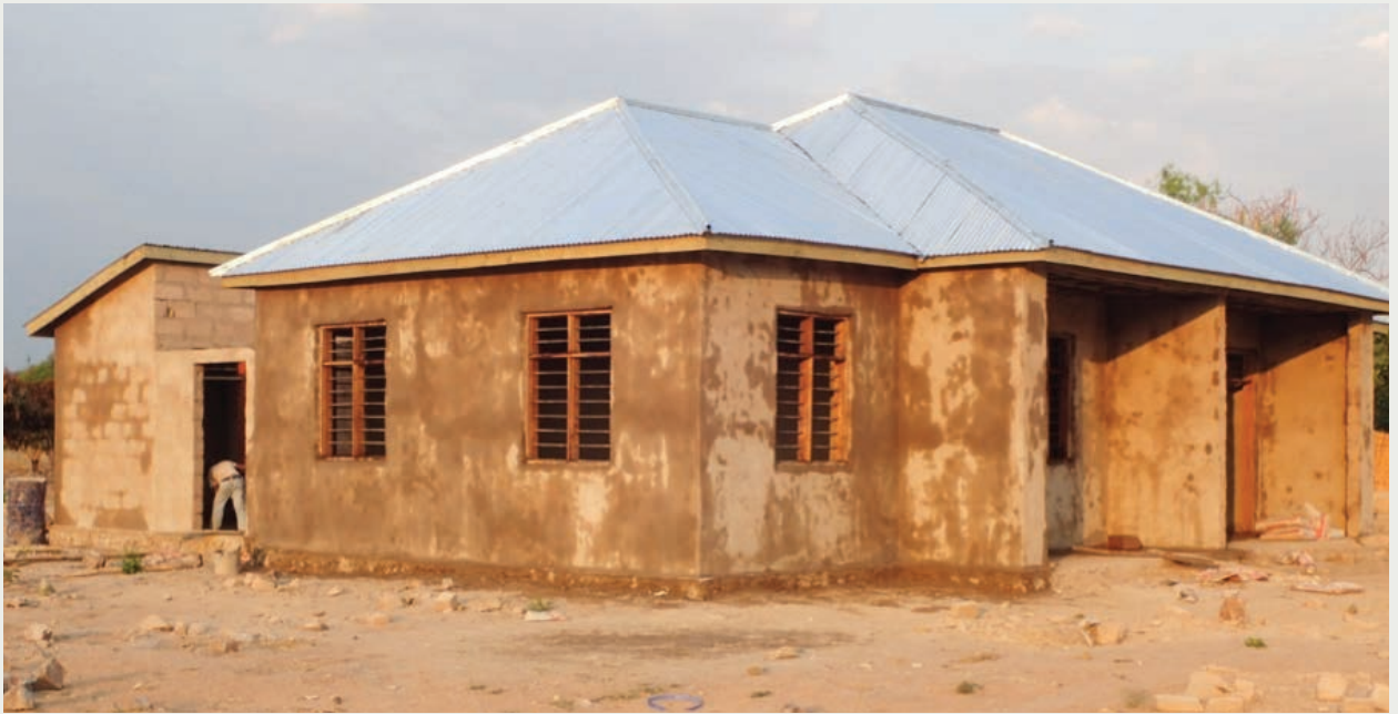
Construction nearing completion on a pair of teachers houses at the Itiziro village, September 2015.
