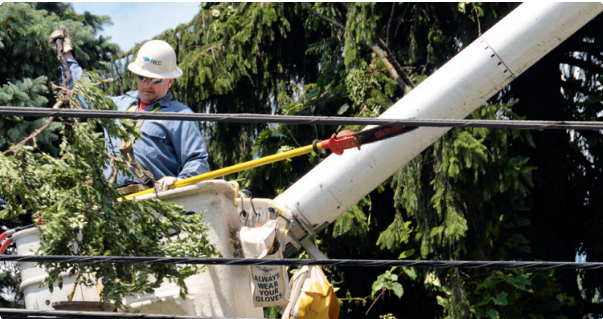
Both ComEd and PECO kept the lights on and the gas flowing despite numerous severe storms throughout the year. This PECO line employee works to safely remove fallen branches from power lines after a summer storm.
