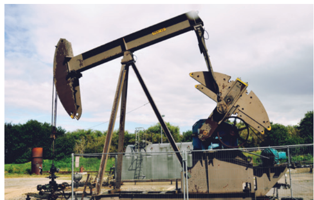
West Firsby #9 well producing on beam pump
