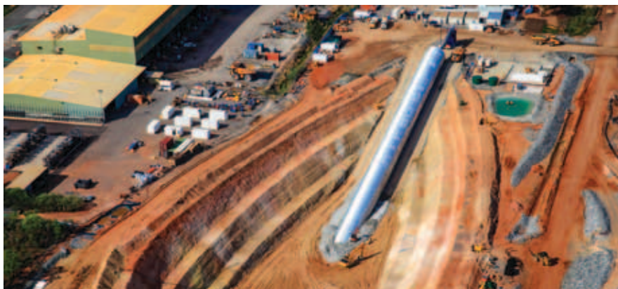
Ranger 3 Deeps exploration decline portal backfill underway in November 2012. The backfill of the box cut was completed in December 2012.
