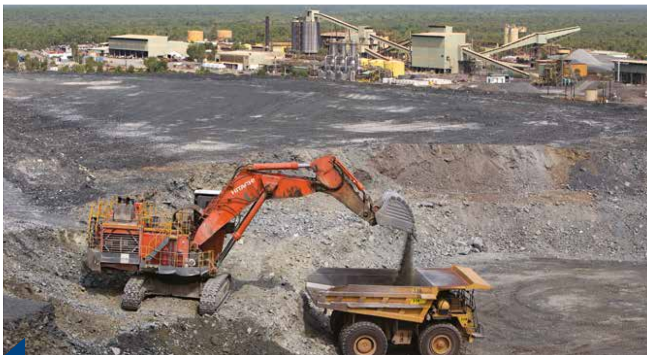
Stockpiled ore is loaded onto a haul truck at Ranger mine, with the processing plant in the background.
