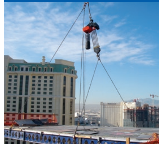
Shown here in Las Vegas, Nevada, the CM Compensator is a 15 ton CM PowerStar Electric Chain Hoist attached to the hook of a tower crane. The system has been engineered specifically to enable the pioneering "flying deck" high-rise construction technique.
