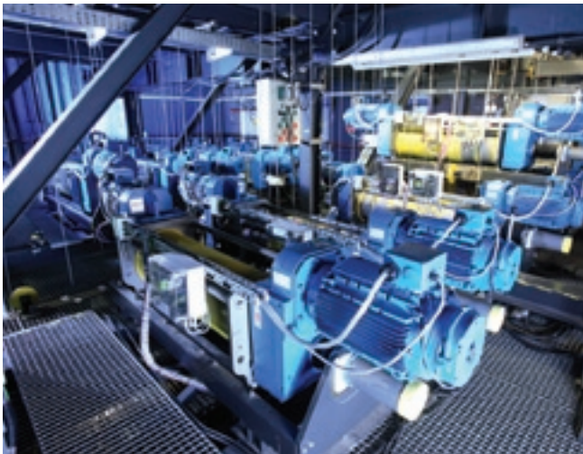
For the Walt Disney Musical TARZAN, the Neue Flora, Europe's largest musical theatre located in Hamburg, Germany, installed Delta electrical wire rope winches in their newly-arranged FlyGrid, including a complete, computerized, control system made by Pfaff-silberblau.
