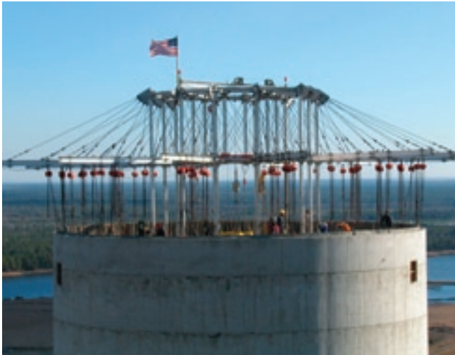
These CM Cyclone manual chain hoists are used to pull concrete formwork on a chimney construction project at a power station in South Carolina. (photo courtesy of Commonwealth Dynamics, Inc., Chimneys, Stacks, Silos, Cooling towers, www.comdynam.com )
