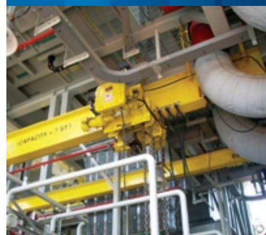
A seven-metric ton capacity, explosion-proof, corrosion-resistant, electric, low headroom chain hoist is used to service a gas compressor on an oil production platform off the coast of Angola, Africa.
