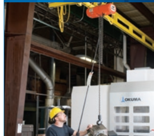
This manufacturing facility in Ohio, USA, uses a CM Lodestar freestanding, enclosed track crane system, with a Lodestar electric chain hoist, to move fixtures and tooling in and out of their CNC machine.
