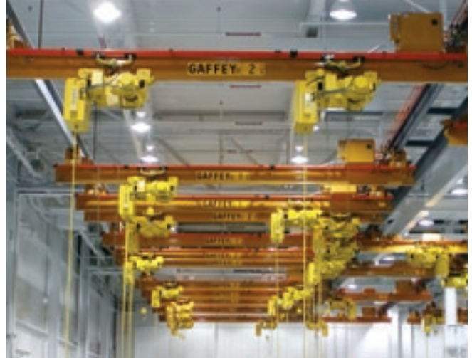
CM's under running, patent track Gaffey cranes are used to interlock 37 bridges, allowing 70 Yale Cable King wire rope hoists to move from one bay to another, providing flexible and flawless handling of the jet engines at this engine repair facility in Texas, USA.
