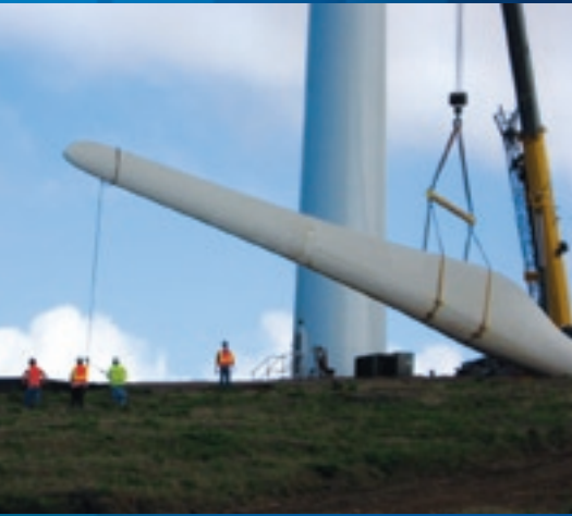
This wind farm installation in Hawaii, USA, uses an extensive rigging system of CM spreader beams, synthetic slings, and shackles to lift the blades, tower sections, hubs, and nacelles into position.
