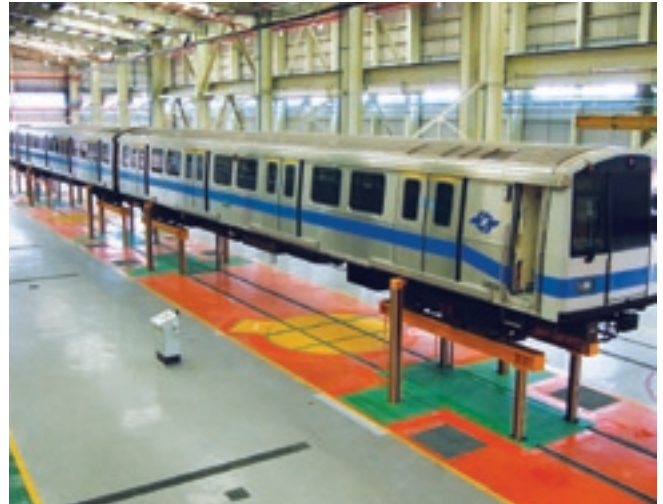
The Pfaff-silberblau 150-ton under-floor lifting system with turntables installation, used by the Taipei Rapid Transit Corporation in Taiwan to lift its trains for maintenance, is earthquake resistant.
