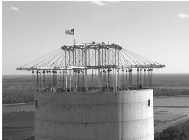
70 CM Cyclone hand chain hoists are used during the construction of a reinforced concrete chimney at the Santee Cooper Winyah Generating Station in South Carolina.
