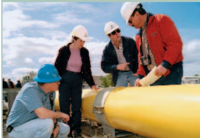
Federal and state regulators work with NW Natural to inspect pipelines for safety. Above (left to right) are Al Jones, pipeline safety engineer with the Washington Utilities and Transportation Commission; NW Natural Design Engineer Jodi Wright and Chief Engineer Bruce Paskett; and Steve Rieger, engineer with the U.S. Department of Transportation, Office of Pipeline Safety.
