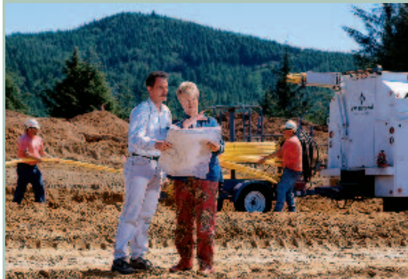
NW Natural’s Lincoln City Utility Coordinator Judy Thompson reviews building plans for the new Summit Ridge subdivision with Dan James, owner of Northwest Homes. NW Natural works closely with builders to coordinate construction and ensure the smooth installation of natural gas service.
