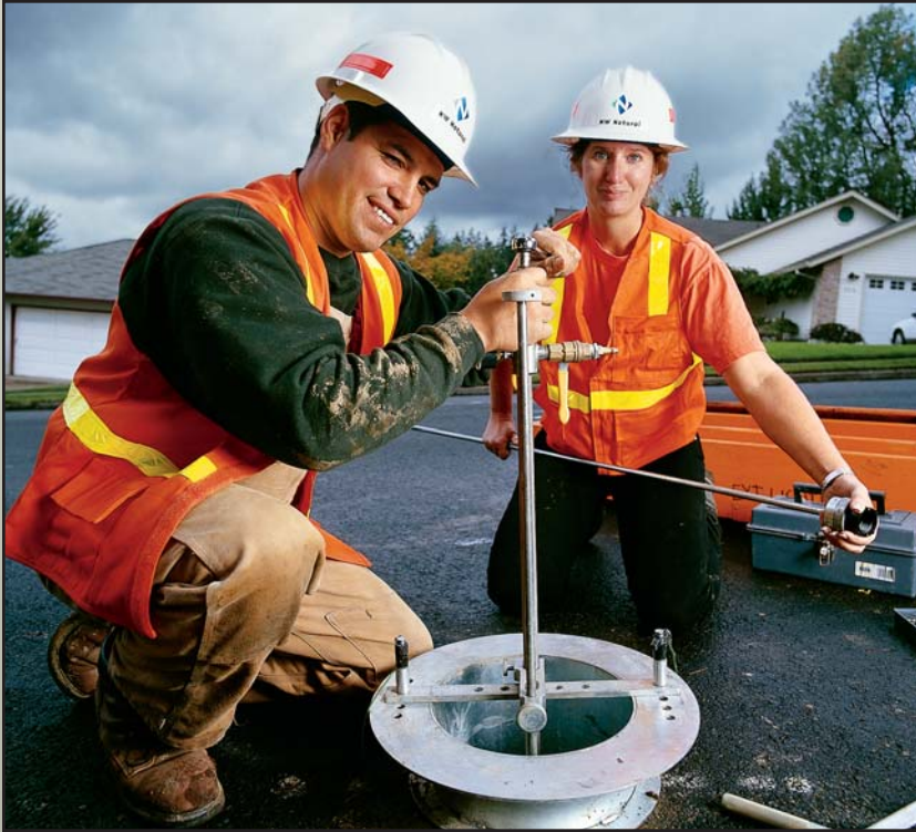
Clark County Distribution Crew Leader Clark Apodaca and Pipe Joiner Wendy McDowell install a new residential service using keyhole technology pioneered by NW Natural.
