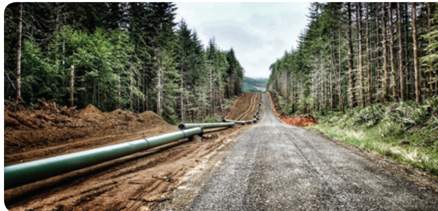
➤ Construction of the 16-inch portion of the pipeline for the North Mist Expansion project is complete.
