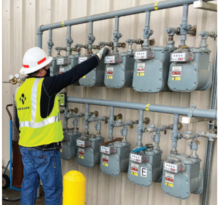
NW Natural technicians testing blended hydrogen gas at NW Natural's Sherwood facility.
