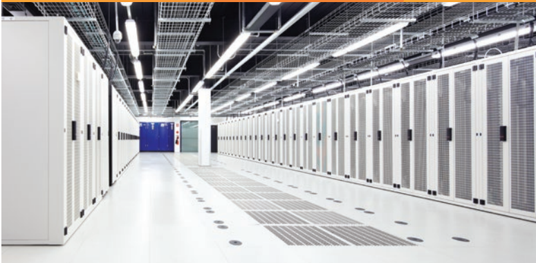
> Macquarie Telecom Data Centre, Sydney Australia
