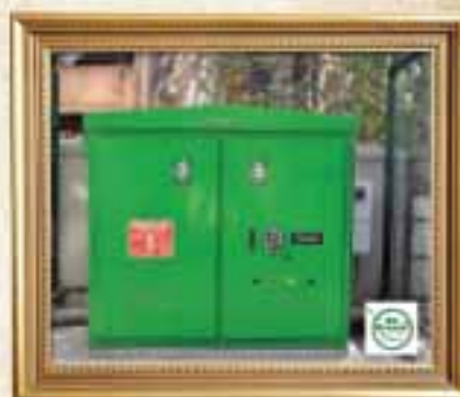
India's first Green, Safe and Compact Natural Ester based Pad Mount Substation
