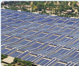
World's largest solar rooftop installation of 12 MW for RSSB-EES, Amritsar (single location, multi-roof)
