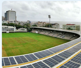
World's largest solar rooftop installation on a cricket stadium of 820.8 kWp at Cricket Club of India, Mumbai
