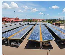
India's largest solar carport of 2.67 MW at Cochin International Airport Limited (CIAL)
