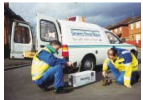
Severn Trent Water engineers installing Palmer Environmental's revolutionary Permalog leak detection system. Data from permanently fitted underground sensors is collected remotely from a passing vehicle.
