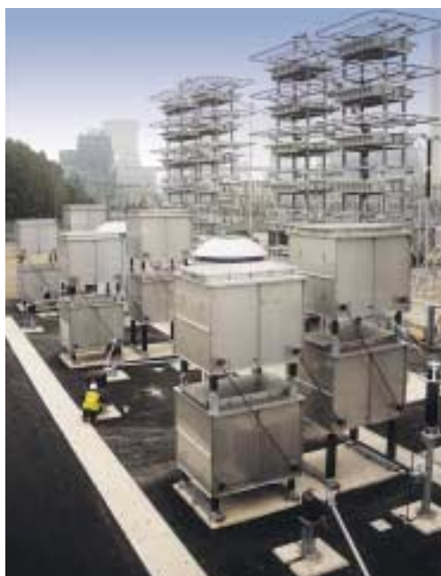
Cressall filter resistors improve power transmission efficiency at the Willington Power Station, England.
