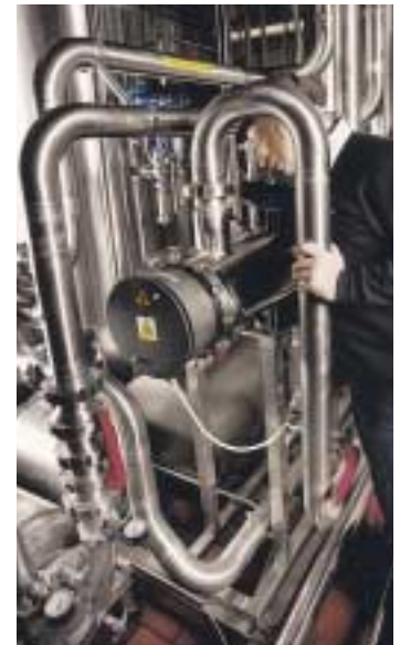
One million litres of water per day for soft drinks production is treated by Hanovia UV systems at the Silver Spring Mineral Water Company, England.
