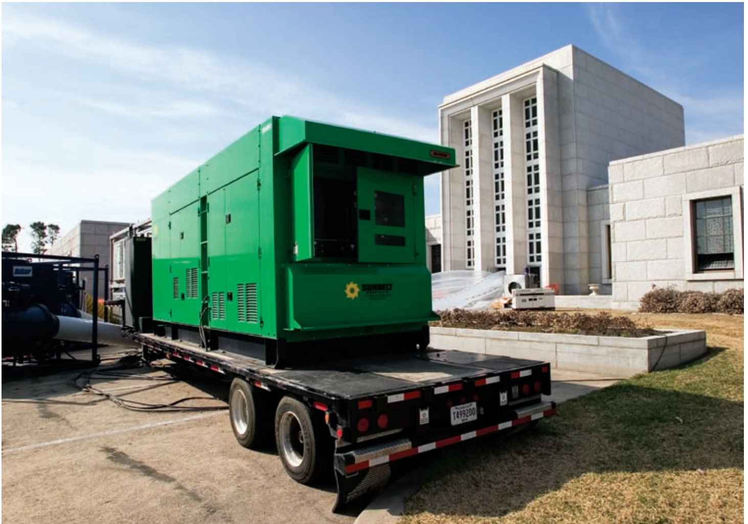
Sunbelt's diesel-driven generators provide emergency power for diverse needs.
