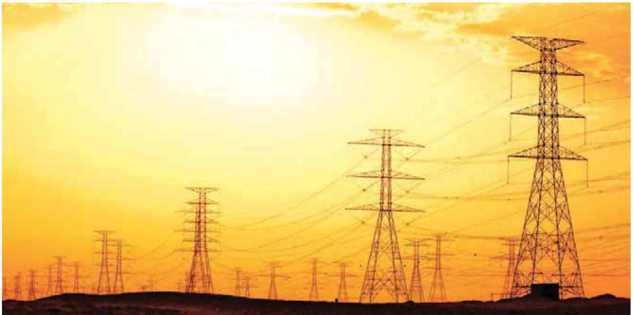
230 kV double-circuit transmission line at Abu Ali, Saudi Arabia. L&T is the industry leader in turnkey construction of power transmission and distribution systems in India and the Middle East.
