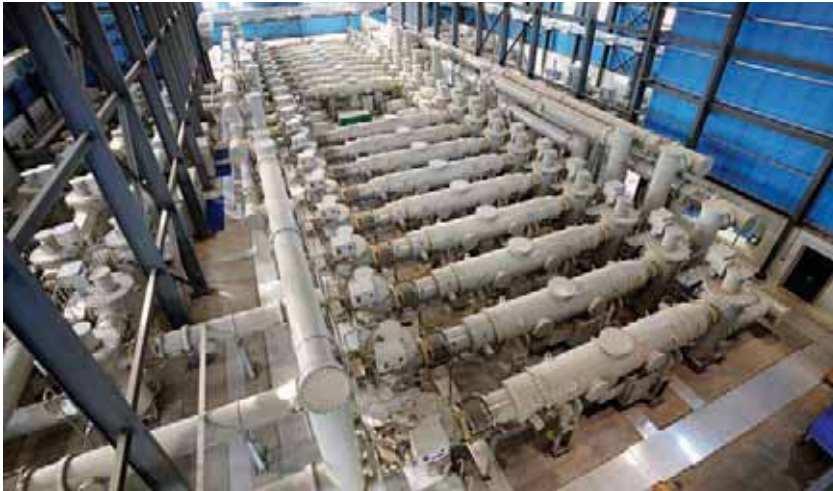
India's first 765 kV Gas-insulated Substation, at Pune.
