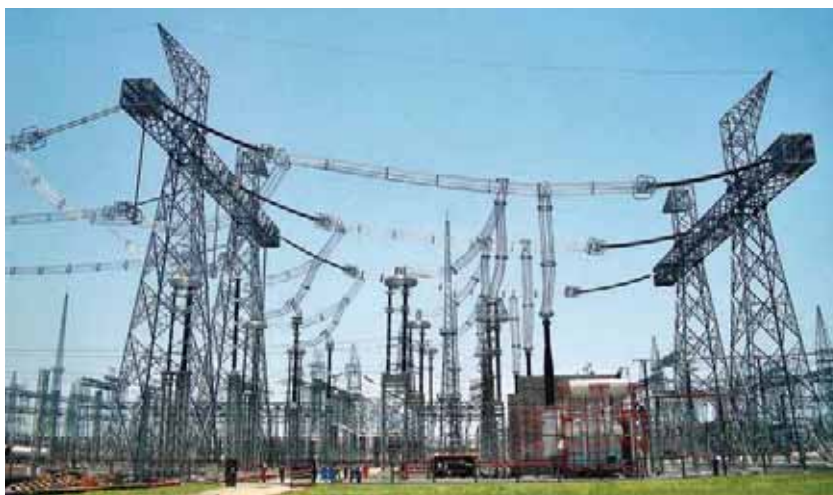
India's first 1200 kV Air-insulated Substation at Bina in Madhya Pradesh.
