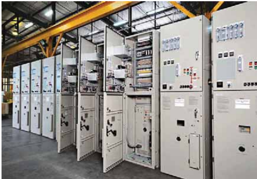
Switchboard installation at a power plant. L&T provides power distribution and control solutions across the value chain, from generation to end user.
