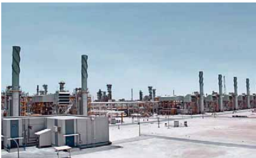
Upgrade project executed on an EPC basis for export gas compression facilities of Dolphin Energy, Qatar.
