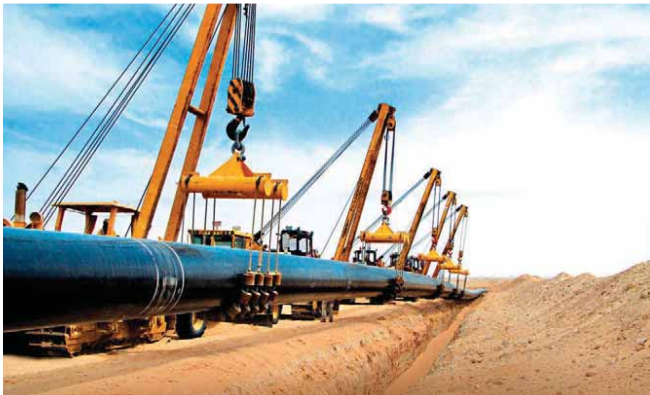
Habshan-Ruwais-Shuweihat gas pipeline project built on an EPC basis for GASCO, Abu Dhabi.
