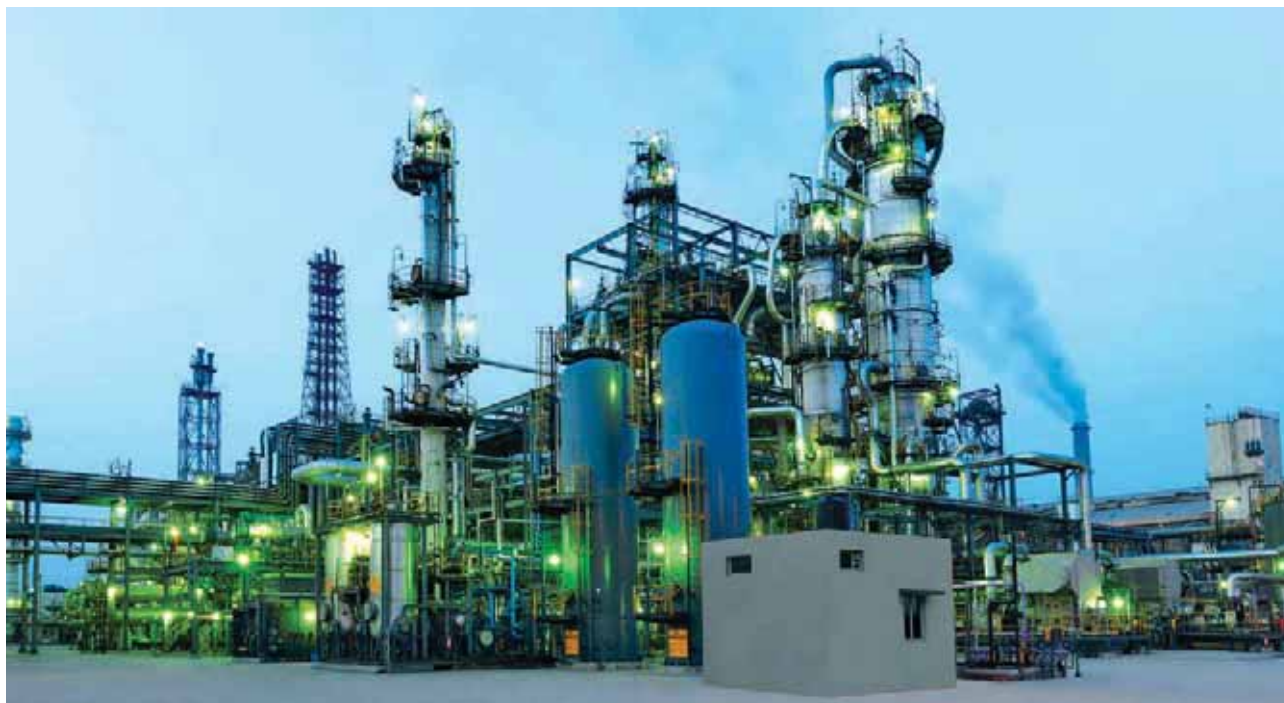
900 TPD Ammonia plant modernisation project for National Fertilizers Limited - one of many onshore projects executed on a License+EPC basis.
