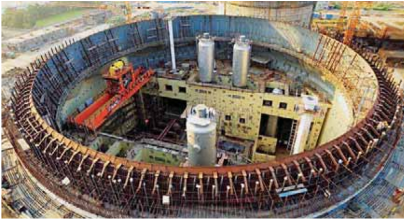
L&T is building the Kakrapar Nuclear Power Plant in Gujarat - the latest in its 5-decade association with India's nuclear power programme.
