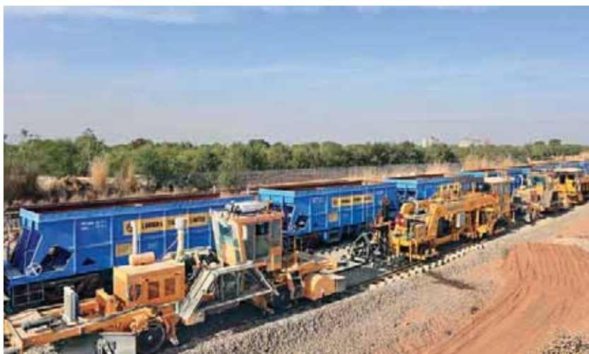
The new track construction machine is capable of laying 2 km of tracks per day, setting a benchmark in high-speed rail construction on the Western Dedicated Freight Corridor project.
