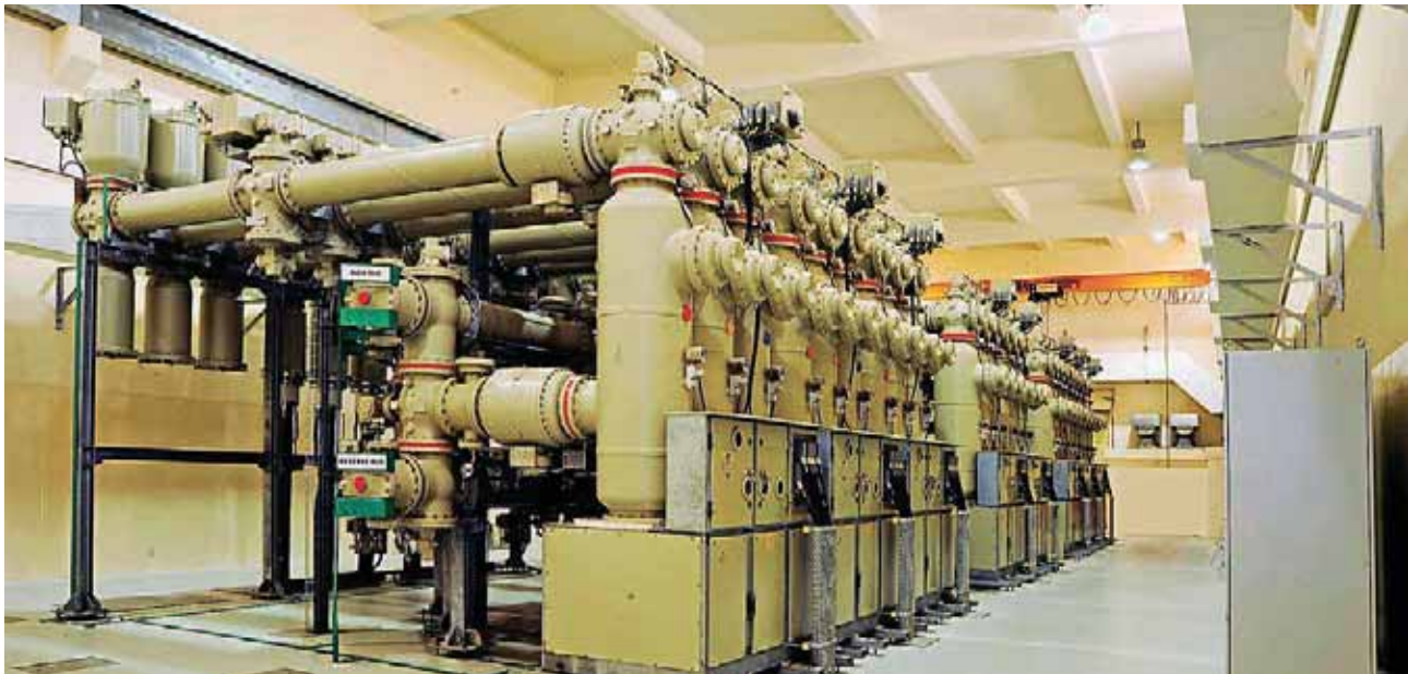
One of the many 400 kV Gas-insulated Substations installed by L&T.
