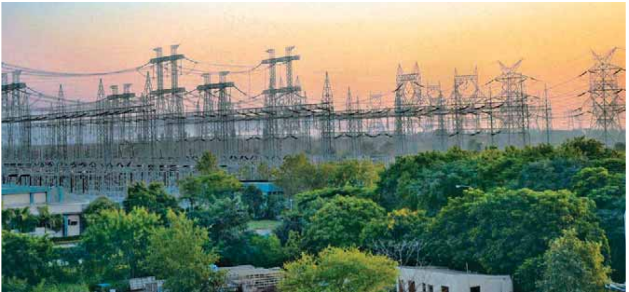
L&T's capability in executing projects for power distribution includes switchyards.
