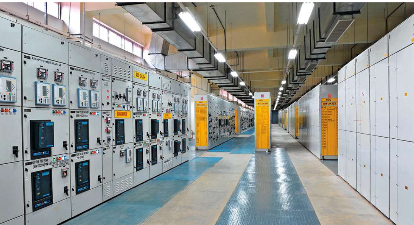
Switchboard installation at a power plant. L&T provides power distribution and control solutions across the value chain, from generation to end user.
