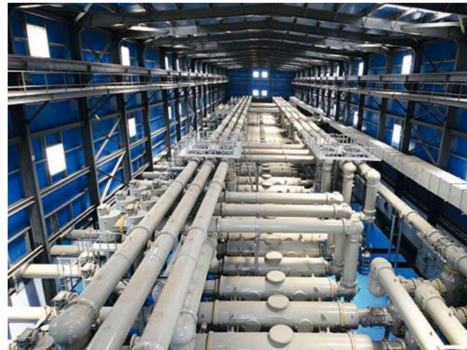
765 kV Gas-insulated Substation, Varanasi.
