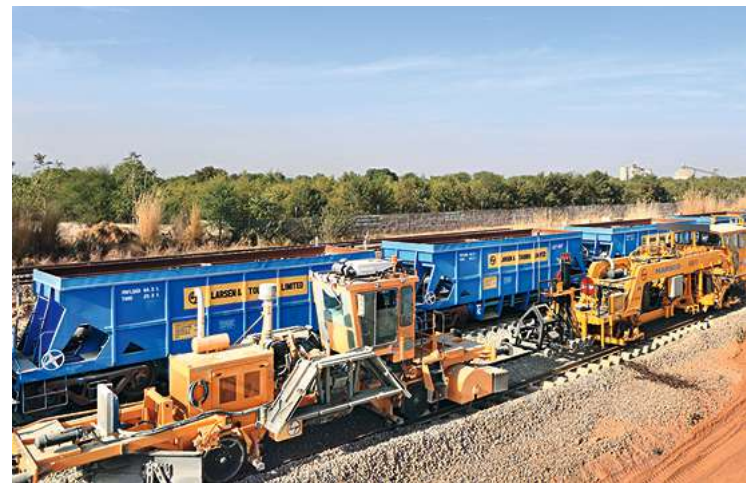
L&T has deployed a new track construction machine capable of laying 2 km of tracks per day - setting a benchmark in high-speed rail construction.
