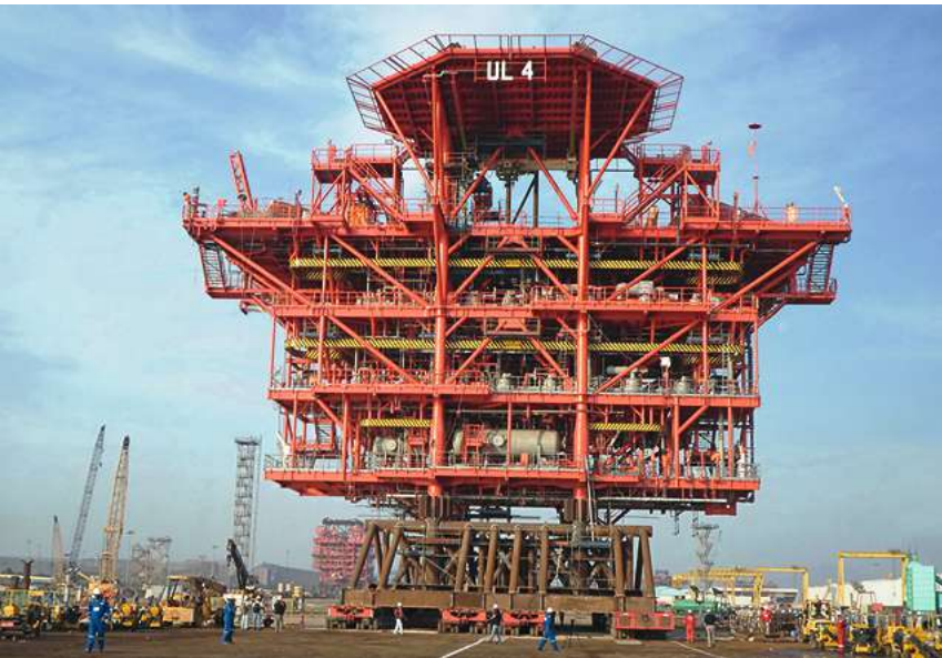
Load-out of offshore modules for ADMA-OPCO, Abu Dhabi from Sohar Yard in Oman
