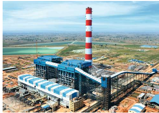
First supercritical coal-fired power project (full EPC) by L&T for Nabha Power Ltd. at Rajpura in Punjab.
