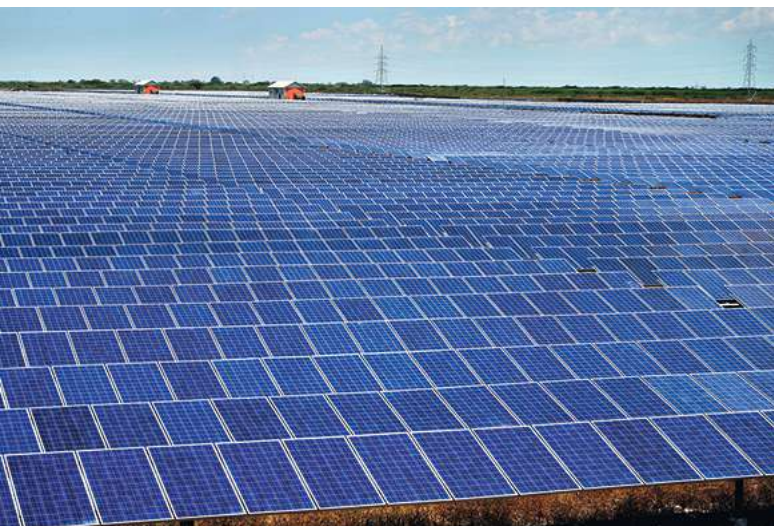
60 MWp Solar Tracker Plant, Tamil Nadu
