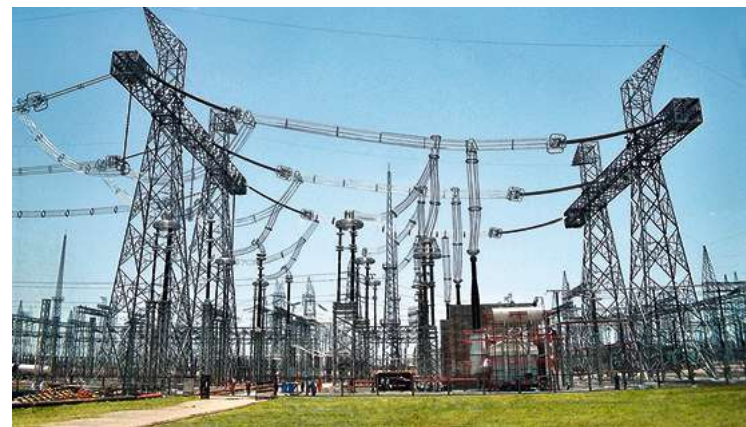
India's first 1200 kV Air-insulated Substation at Bina in Madhya Pradesh.
