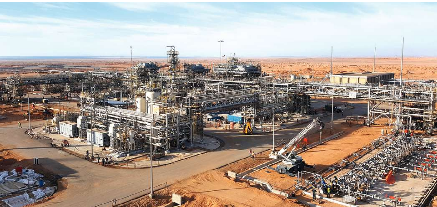
Gas processing facilities for Saudi Aramco near Tabuk in Saudi Arabia.
