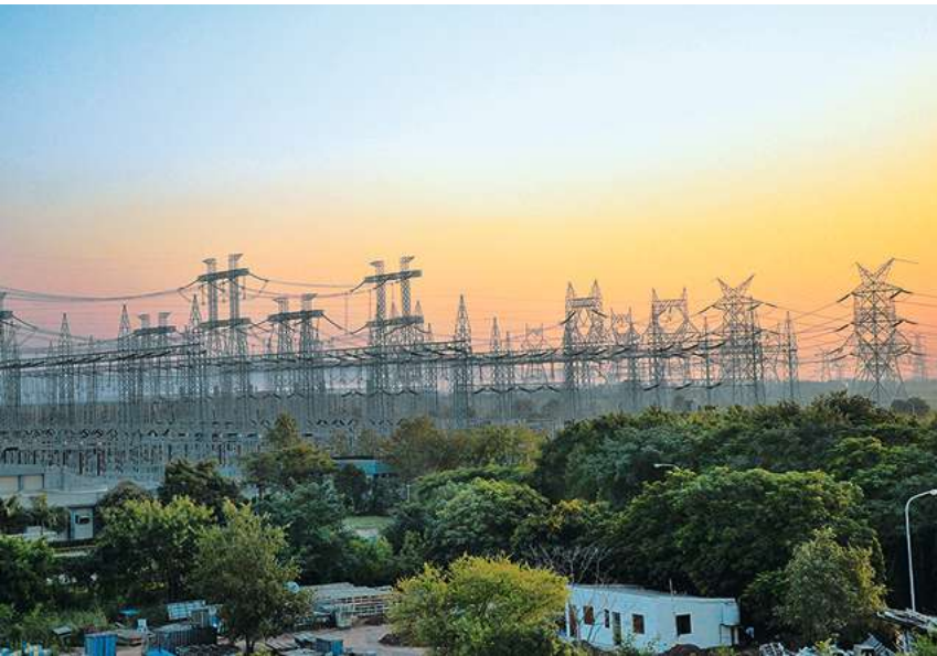
L&T's capability in executing projects for power distribution includes switchyards.
