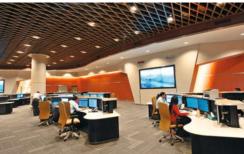
Mumbai International Airport's Network Operations Centre – powered by L&T's Control and Automation solutions
