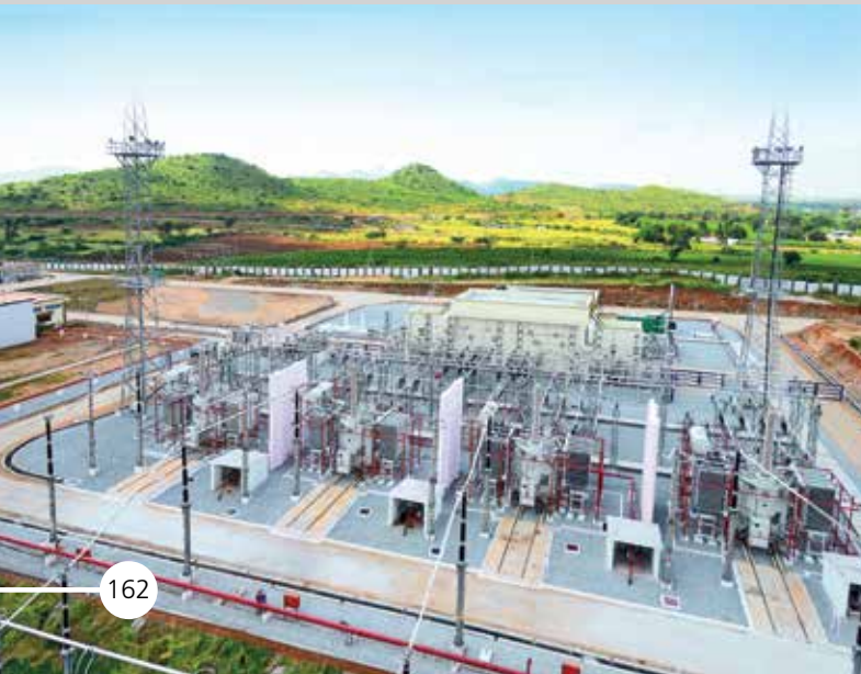
100 MVAR STATCOM at 400 kV NP Kunta Substation, Andhra Pradesh
