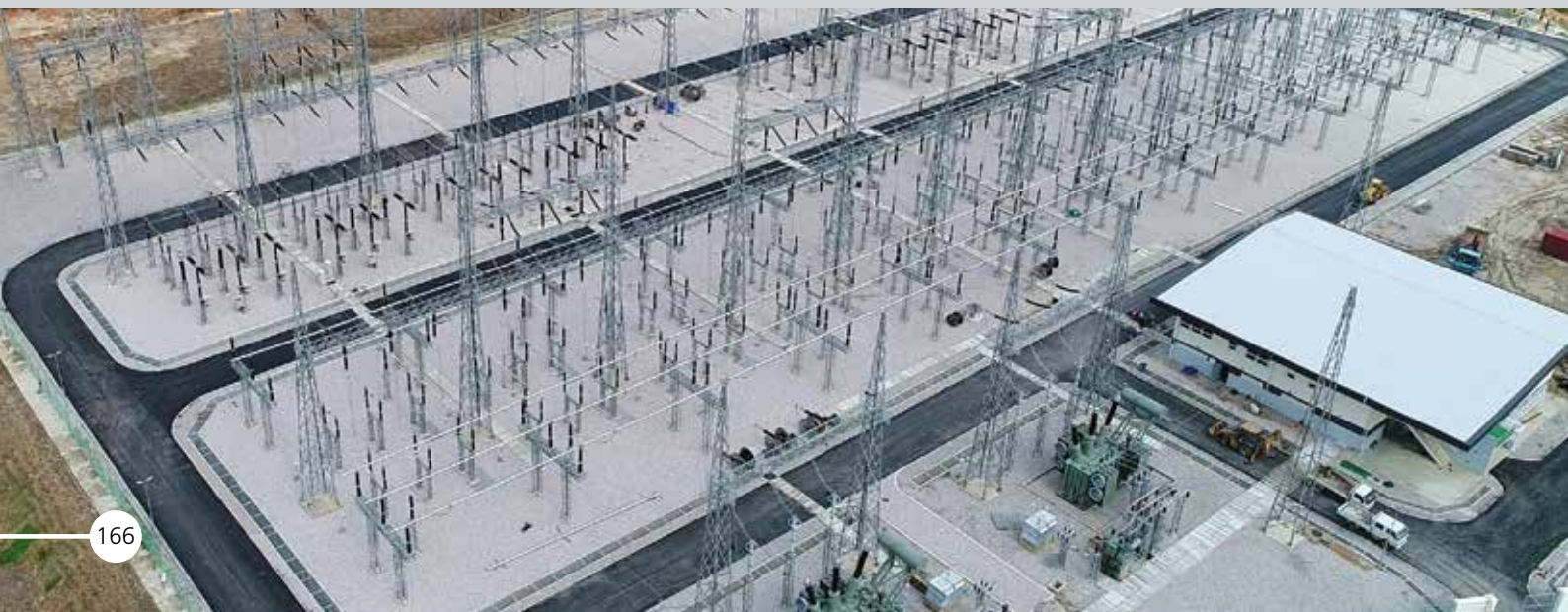
275 kV Air Insulated Substation at Lambir, Malaysia
