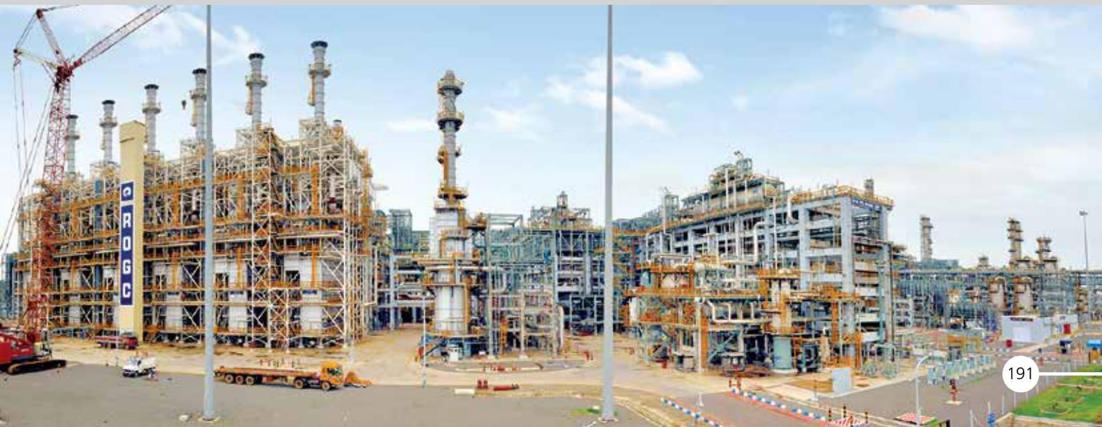
Major role in construction of world's largest Pet Coke Gasification Complex and Ethylene cracker for Reliance Industries at Jamnagar, India
