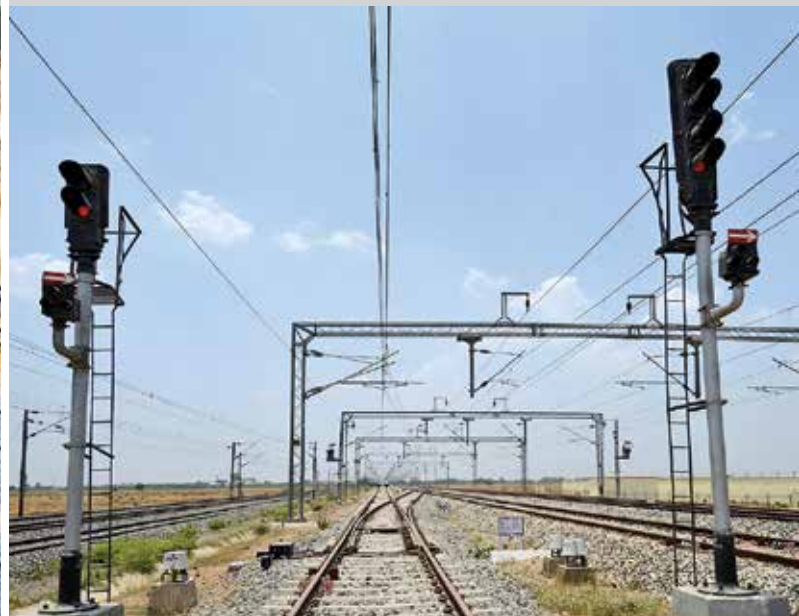
Railway Signaling & Telecommunication
