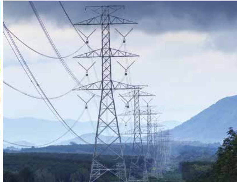
500 kV Tha Li-Khon Kaen 4 Transmission Line, Thailand
