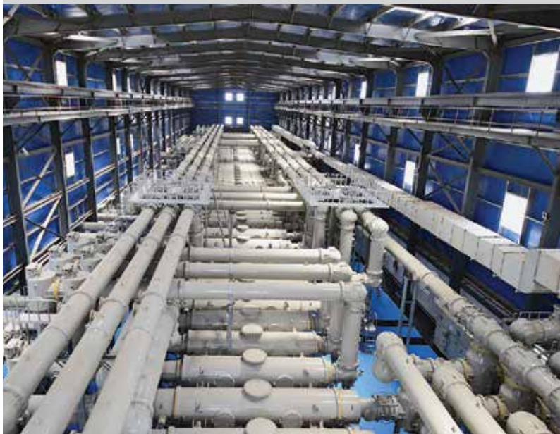
756 kV Gas Insulated Substation at Varanasi
