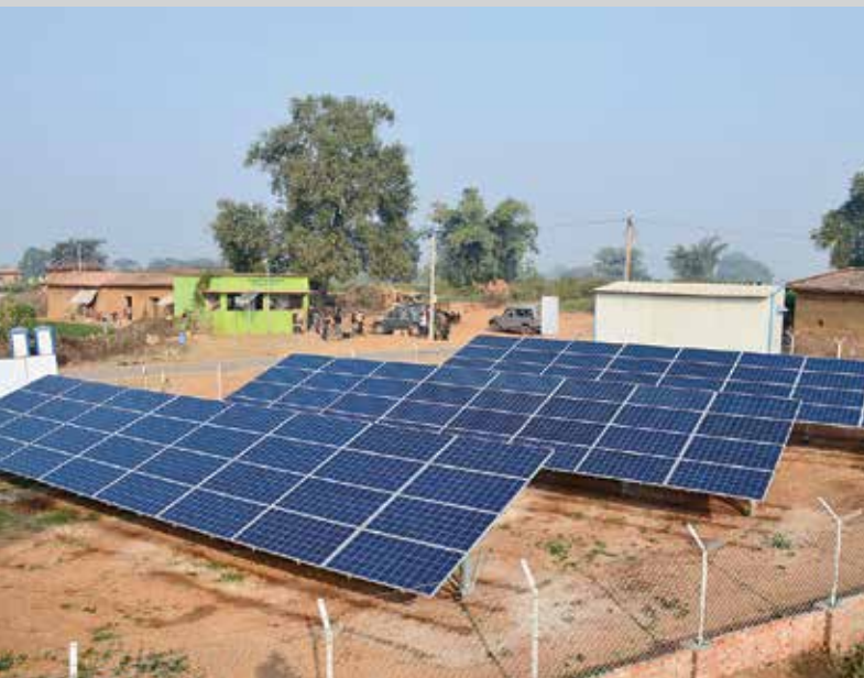
Microgrid Project for Rural Electrification in Bihar
