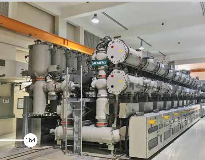
220 kV Gas Insulated Substation at Mehairja, Qatar
