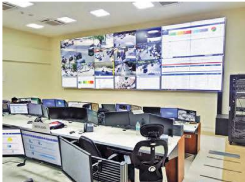
City Command & Control Centre, Vadodara Municipal Corporation.
