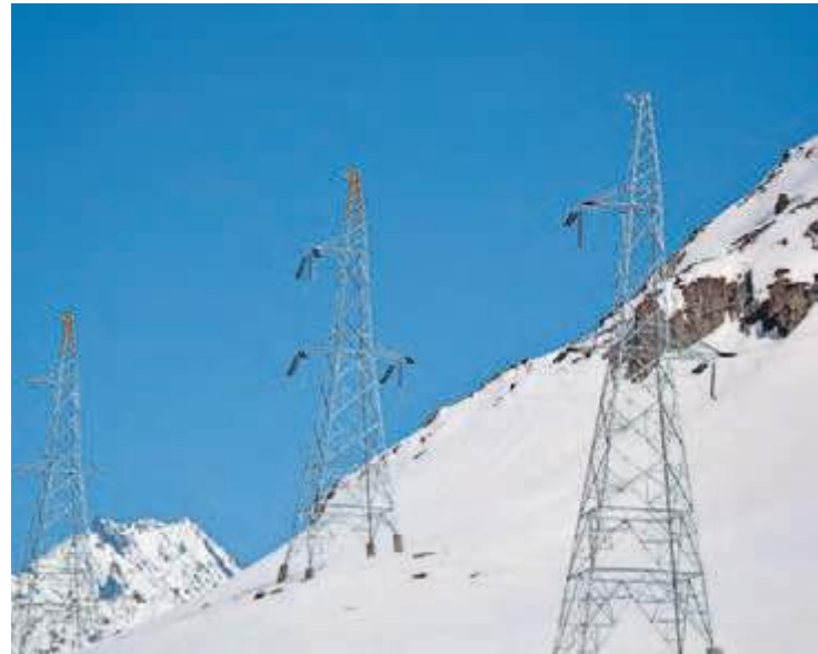
220 kV Alusteng-Drass Transmission Line, Jammu
