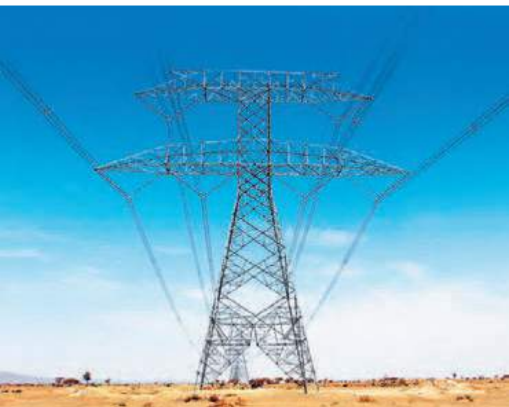
400 kV Ibri-Izki Transmission Line, Oman
