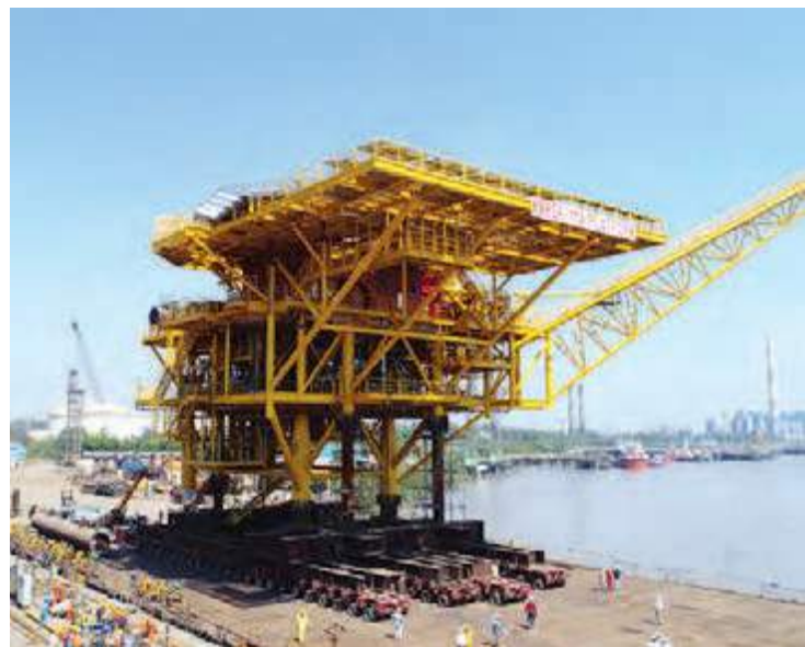
Load-out of BSE-11A Topside for Bassein Development 3 Well Platform & Pipeline Project of ONGC from Modular Fabrication Facility at Hazira, India
