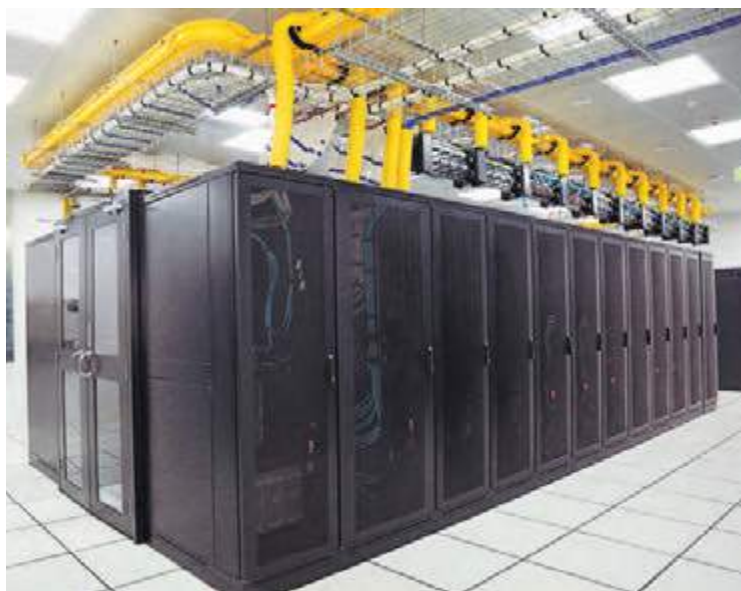
Data Center, Hyderabad
