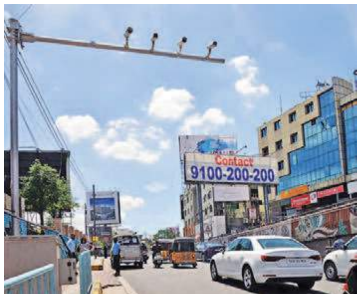
Intelligent Traffic Management System at a critical junction, Hyderabad
