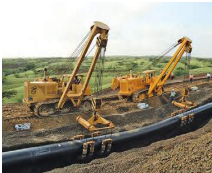
Laying of 36" x 67 km-long natural gas pipeline from Anjar to Mundra in Gujarat for Gujarat State Petronet Limited on EPC basis
