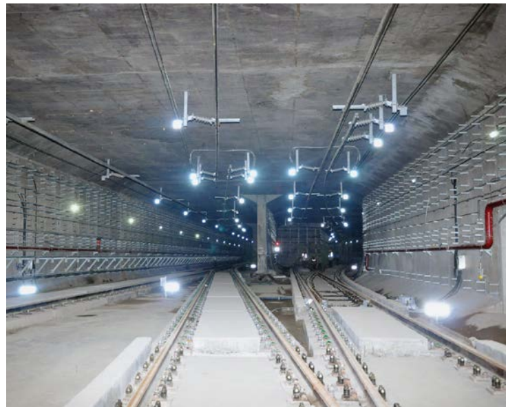
Rigid Overhead Contact System in Phase 3 Tunnel, Delhi Metro
