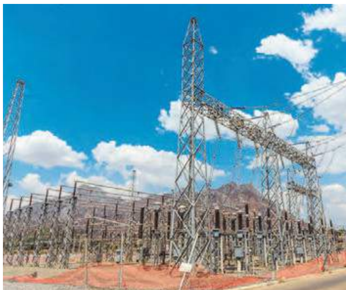
400/132kV Substation, Nkhoma, Malawi
