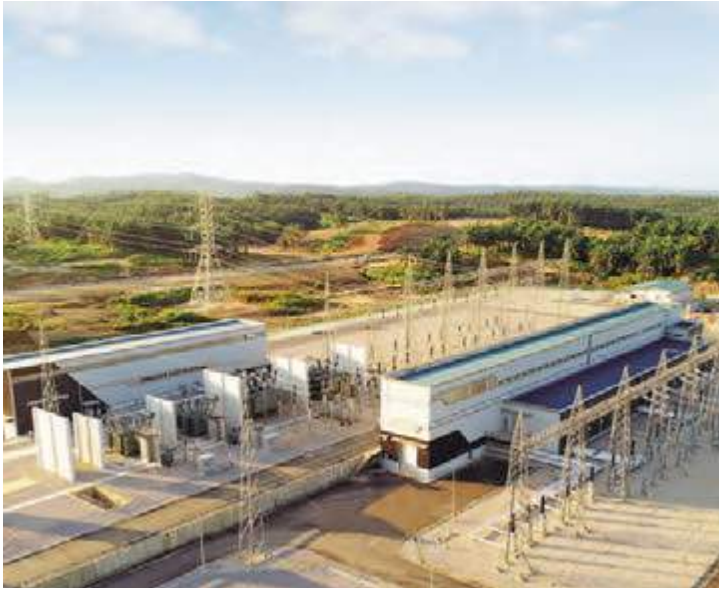
275/132/33kV Gas Insulated Substation, Samalaju, Malaysia
