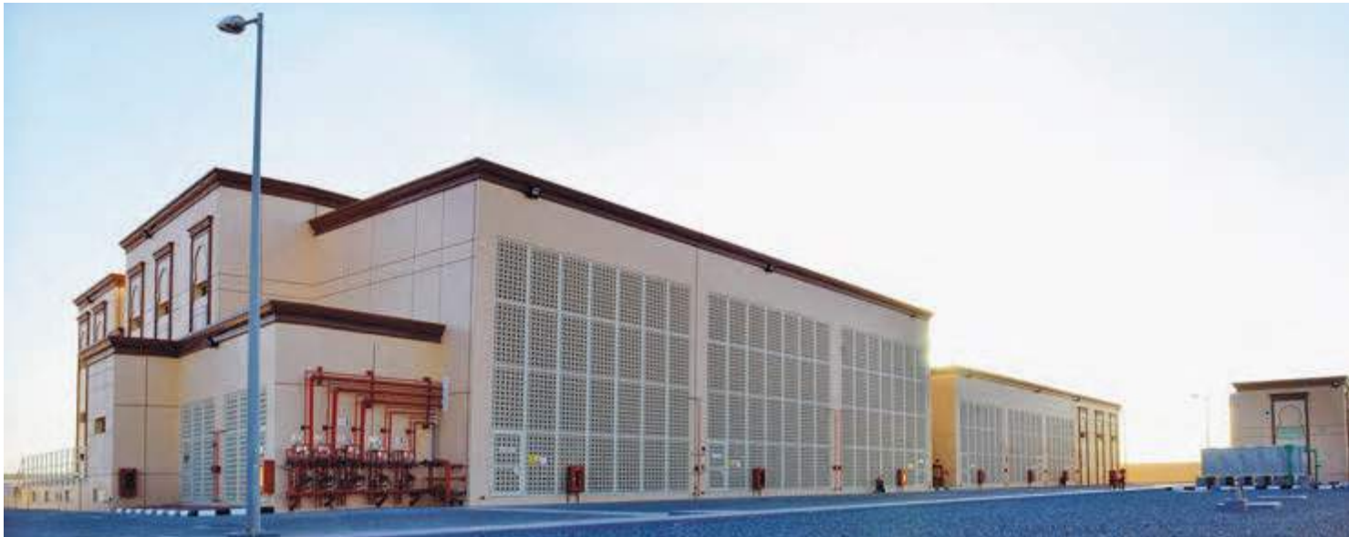
132/33/11kV Substation, Umm Al Quawain, UAE
