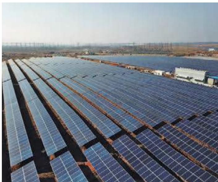
250 MW Solar PV Plant at Rewa, Madhya Pradesh
