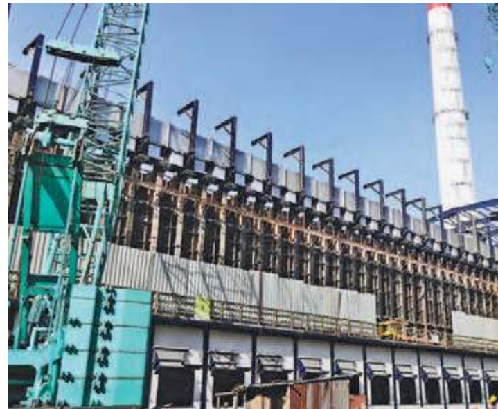
Coke Oven Battery
