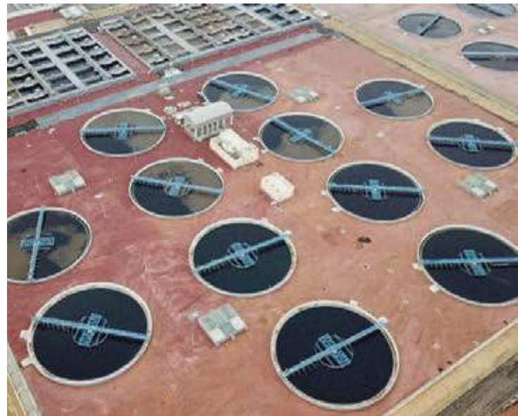
375 MLD Sewage Treatment Plant at Jebel Ali, UAE
