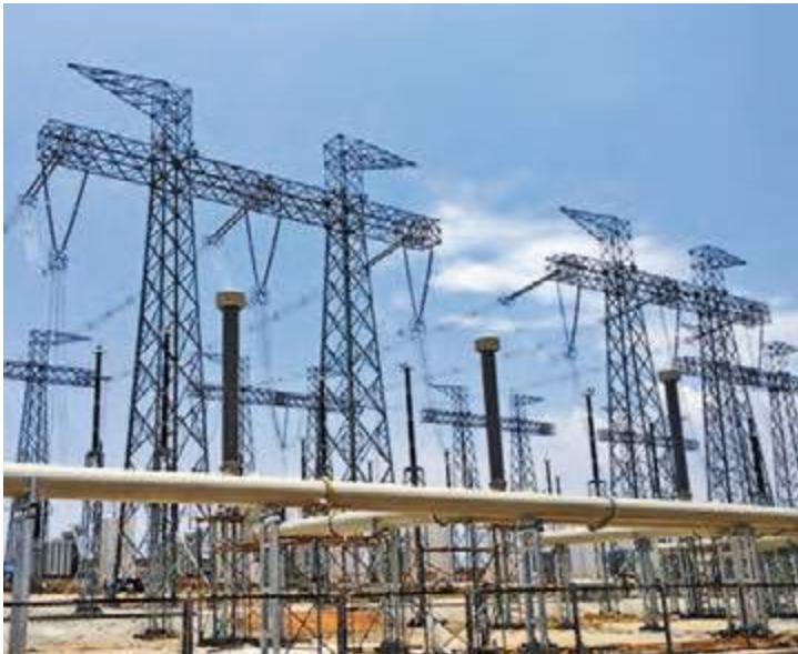
765 kV Gas Insulated Substation, Hyderabad
