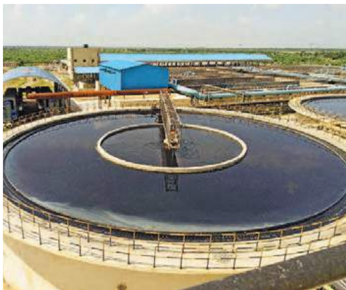
Common Effluent Treatment Plant, Narol
