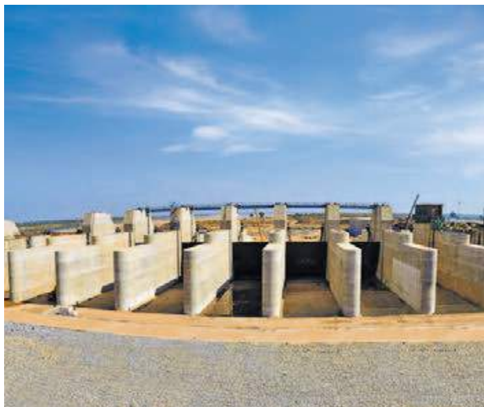
Medigadda Barrage Project, Telanaga - a part of the world's largest multi-stage lift irrigation project
