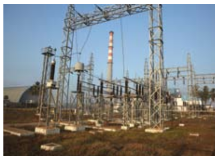
Chennai Plant Switch Yard
