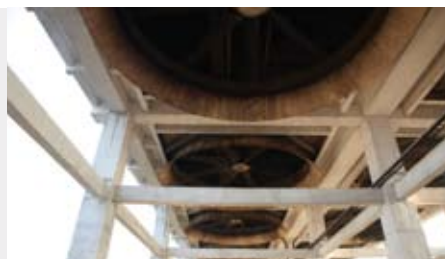
Chennai I Air Cooled Condenser
