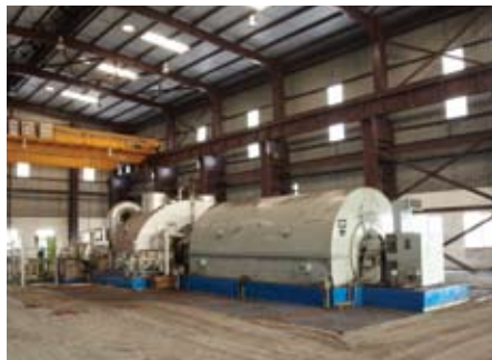
Turbine of Chennai I
