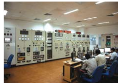
Chennai I Control Room
