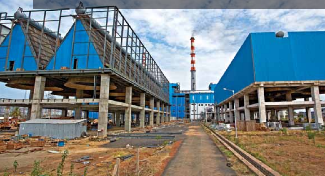
View of Chennai I (right) and Chennai II (left)
