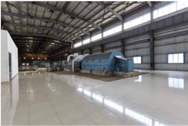
Turbine of completed Chennai II
