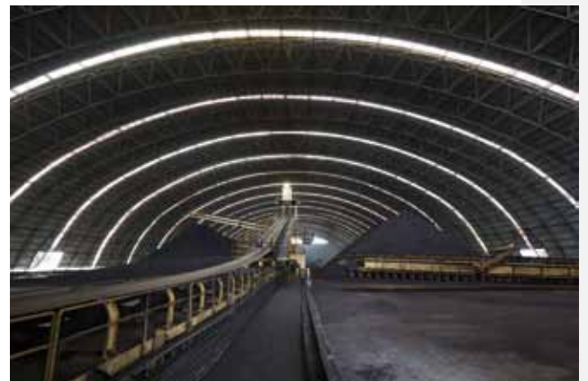
Coal conveyor and stacker at Chennai site
