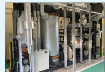
Biomass boiler at Ibaraki Plant
