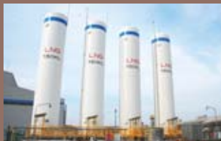
LNG Satellite Terminal (Chiyoda Koshu Co., Ltd.) (Photo: Courtesy of Furukawa-Sky Aluminum Corp.)
