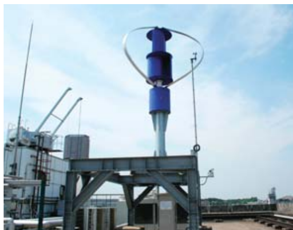
Wind Power Generation Facility at Koyasu Office & Research Park
