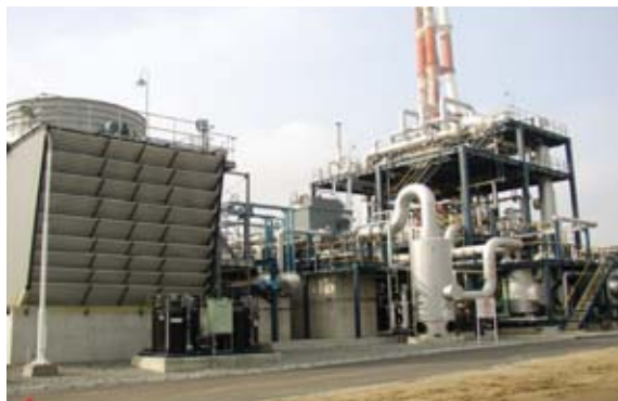
CO 2 and Cold Energy Recovery Unit (Photo: Courtesy of Nippon Petroleum Refining Co., Ltd. and Mitsubishi Chemical Corporation)
