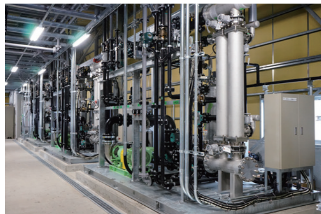
Yabase oil field produced-water treatment verification plant
