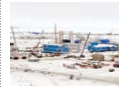
2014 Order awarded for Yamal LNG Project in Russia
