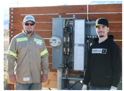
Two university students part of the Maintenance Training Co-operative program assisted in connecting a new generator to the power grid at Florida Canyon.
