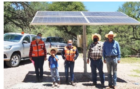
Installing new solar panels at La Cruces and Mimbres ranches near San Agustin.
