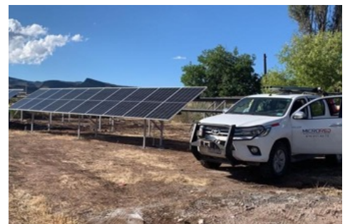
Solar panels installed to provide power for water well pumps in the community of San Lucas, Mexico
