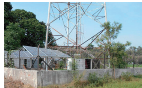
Demonstration Project for Telecom Tower Sites in India
