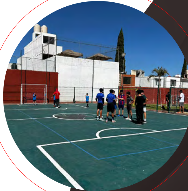
Rehabilitation of a sports facility in Morelia, Mexico, undertaken through a collaborative effort with Fundación Placemaking México.
