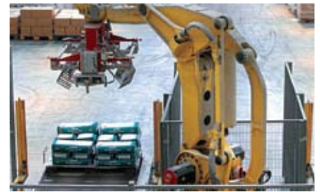
Robotic palletiser stacking product for despatch at the Norcros Adhesives UK manufacturing base.
