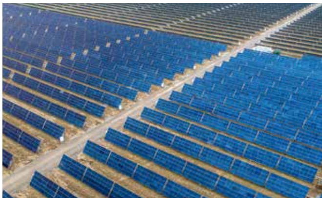
Solar panels at Silicon Ranch, West Virginia, USA.
