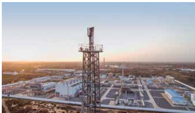
Changbei Natural Gas Processing Facility, China.
