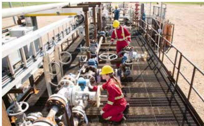
The Quest CCS facility in Alberta, Canada.
