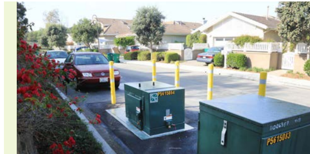
Storing Energy Locally: Batteries can be used locally in homes and neighborhoods to store energy from customers’ distributed generators, such as in this neighborhood in Irvine where these transformers sit atop underground batteries.
