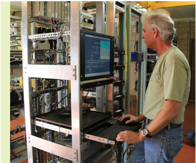
Building a Smarter Grid: Distributed energy is an important component in building the smarter electricity grid of the future, exemplified by this technologically advanced substation in Irvine.
