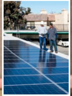
Solar panels on carport roofs.
