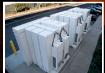
Tesla Energy lithium ion batteries.
