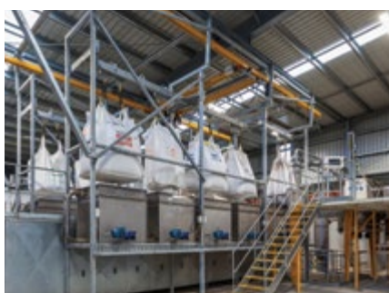
Lara feedmill pre-mix addition area.
