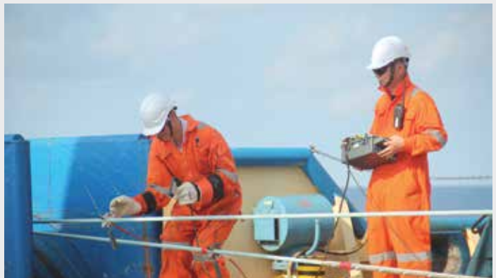
→ December - Indonesia Global Gateway (IGG) Operation , which connects international gateways to the west through SEA-ME-WE 5 and east through SEA-US, was an important milestone for Telkom towards becoming a Global Digital Hub.
