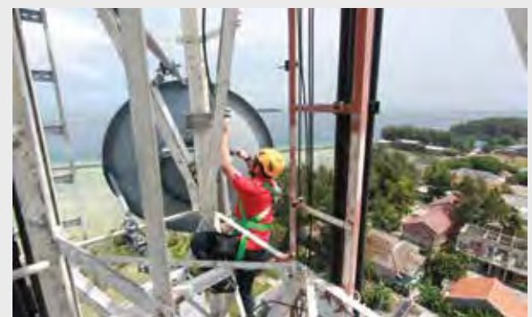
→ December - Telkomsel was getting stronger as the cellular market leader with 189,081 BTS at the end 2018, 73% of which are 3G and 4G BTS covering 90% of the population.
