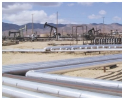
The pipes in the foreground carry (at separate times) both steam to and production from wells at Seneca's Midway-Sunset field in California. These cyclic steaming operations heat the oil reserves, which increases each well's oil producing capability.
