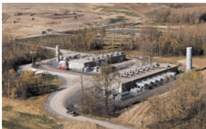
NFR Power owns a 50% interest in this 11.2 megawatt power plant located in Waterloo, New York. This facility generates electricity from methane gas collected from the adjacent Seneca Meadows landfill (in the background).
