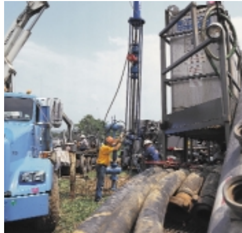
The hydraulic fracturing process increased the injection and withdrawal capabilities of this Supply Corporation storage well near our Nashville Station by fivefold. Pictured above, a temporary valve "stinger assembly" is installed to protect the permanent wellhead and master valve from possible damage from the large volumes of sand and water that are pumped into the well during the fracturing process.
